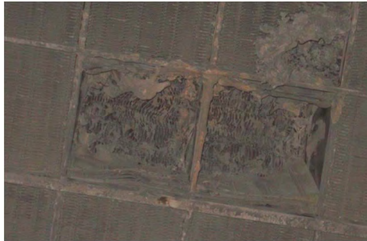
Bottom of Plate Catalyst After Fire Damage
